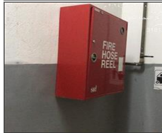
Photo of fire safety equipment FIRE HYDRANT.jpg
