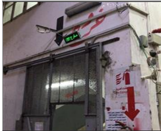
Photo of fire safety equipment EMERGENCY EXIT.jpg
