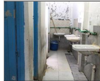
Photo of the sanitary facilities WASHING FACILITY.jpg
