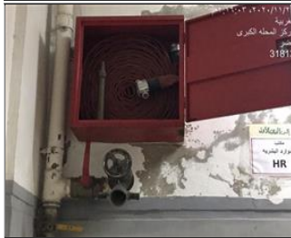
Photo of fire safety equipment FIRE HYDRANT CONTENTS.jpg
