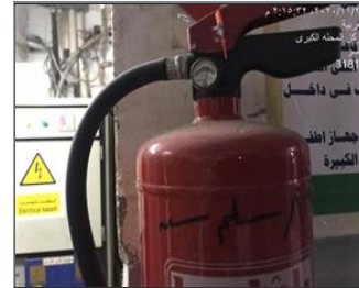
Photo of fire safety equipment FIRE EXTINGUISHERS.jpg
