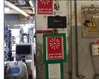
Photo of fire safety equipment ALARM SYSTEM.jpg
