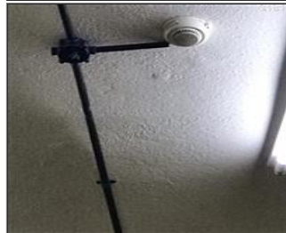
Photo of fire safety equipment Alarm system 2.jpg
