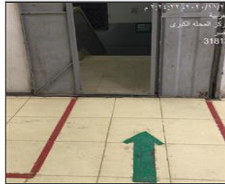
Photo of fire safety equipment EXIT ROUTE.jpg
