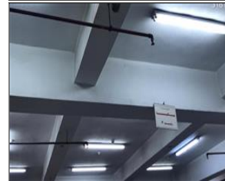
Photo of fire safety equipment sprinklers.jpg
